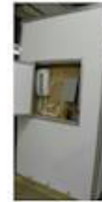
Access Panel 220v Tankless Water Heater.
